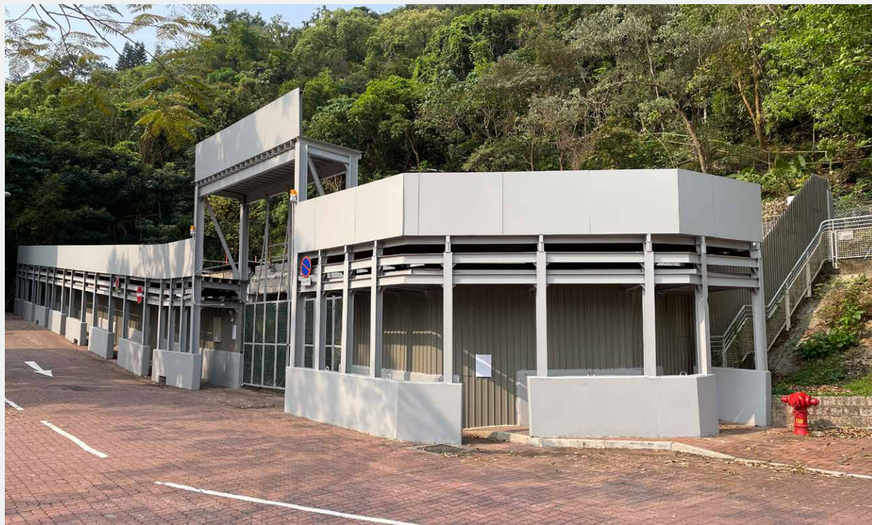
舊教職員宿舍 E 座工地 Construction site of the old Staff Quarters Block E
